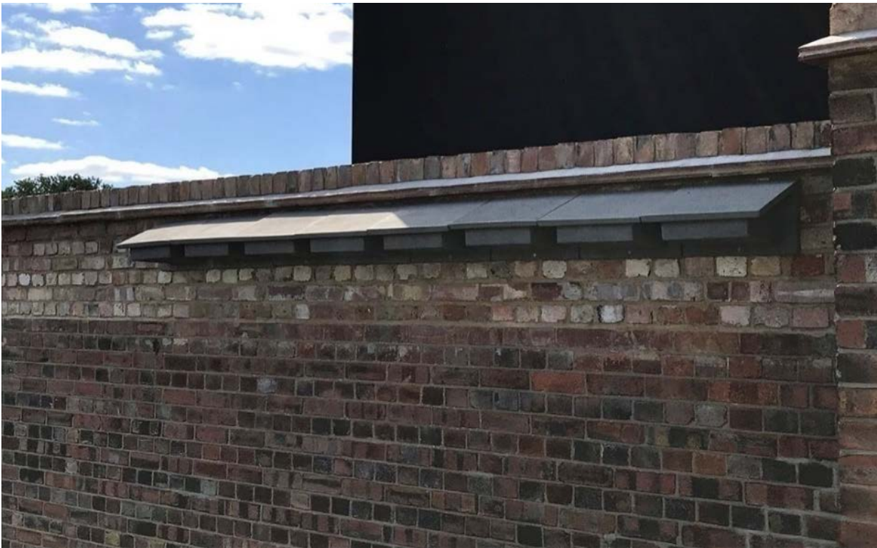
Example of swift boxes in De Beauvoir.
